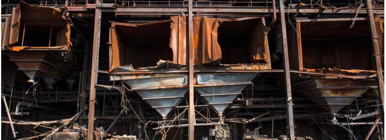
Abandoned plant stands in decay Photographer: Jim Watson/AFP/Getty Images Insights
